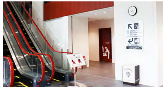
Escalator handrails are in a color that contrasts with the surroundings, making them easy to recognize. Signs are installed in an easy-to-read size.
