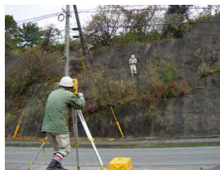
Disaster Prevention Work of Shiratori Housing Complex and Kawasaki Line
