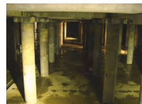
<a facility for storage of rain water>
