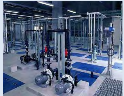
< Exudation water treatment plant >
