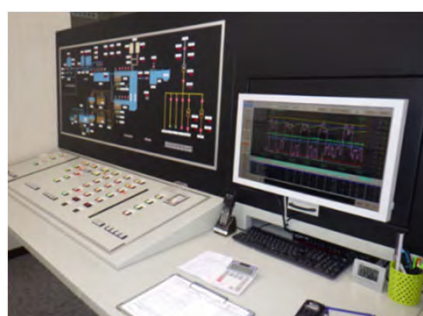
Central monitoring office
