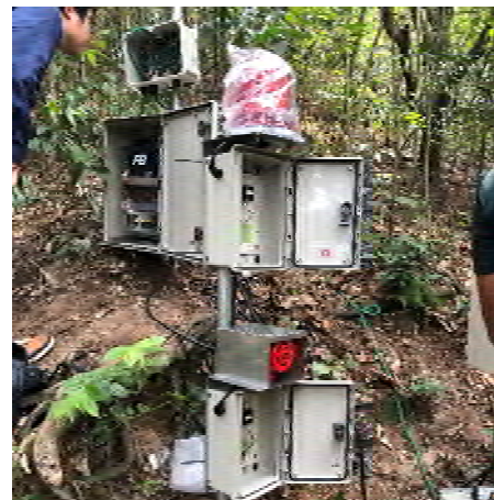
◆ Malaysia Debris flow warning system
