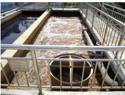
Waste Water Treatment system 1600m 3 /day
