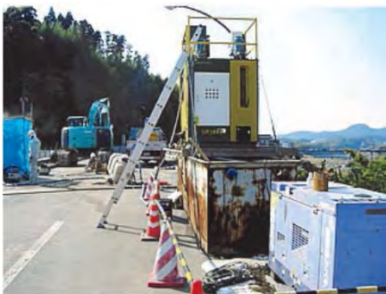
↑ Picture of MLIT project at the construction site Treatment of cutting wastes when dismantle the bridge
