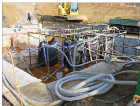
↑ Project picture of Nagano Prefecture’s soil-erosion control office at the construction site. Dredging operations for the Soil-erosion control dam
