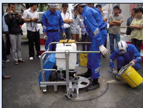
Installation in Dalian, China
