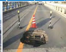
Bridge deck hole
