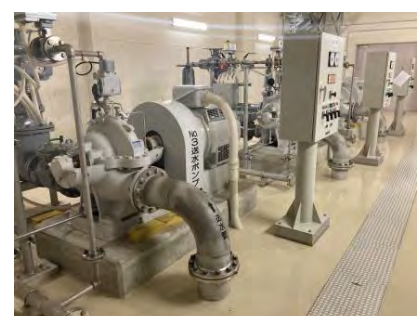
Industrial water pump
