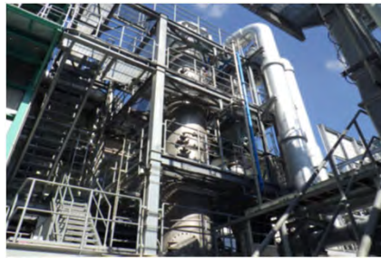
Sewage sludge fuel conversion plant
