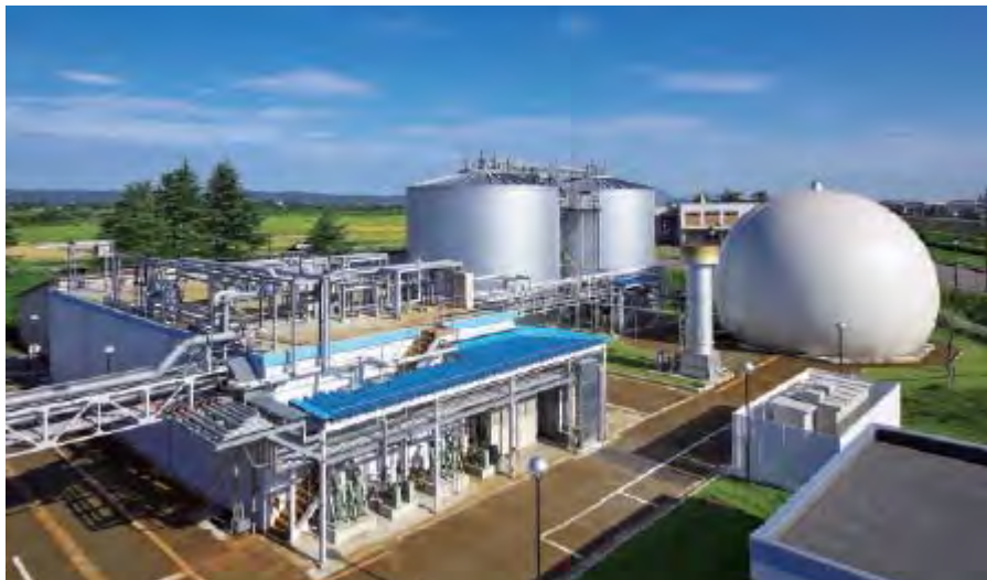
Biomass power generation from kitchen waste (Niigata, Japan)
