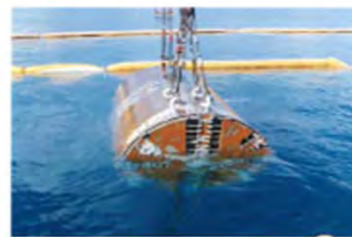
海中からの掘進機の回収 Collecting a tunneling machine from the ocean
