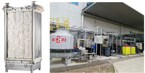
(Left) Membrane Bio-Reactor (MBR) (Right) Zero-Liquid Discharge (ZLD) system
