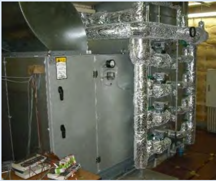
< Cocktail Air-conditioning equipment > (Supply air volume 7,800m 3 /hr)
