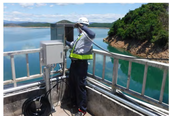
◆ Vietnam Dam gate operation (Gate opening Indicator, Quartz-type water level gauge)
