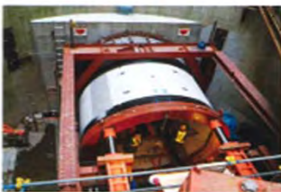
超大口径管の推進状況(発進立坑) The jacking method for the ultra-large diameter pipes is in process (starting shaft)
