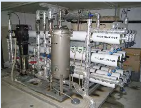
< RO membrane facility >
