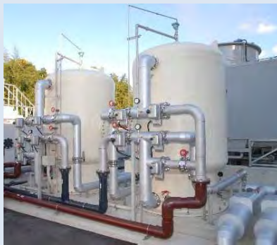
< Sand filtration facility >
