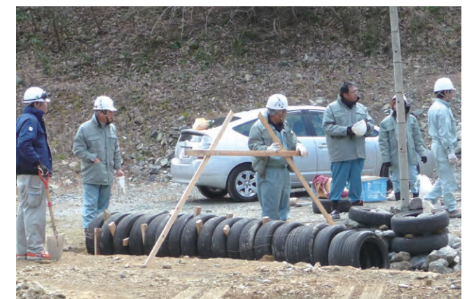
Practical training on installation of leachate collection pipes by use of waste tires.
