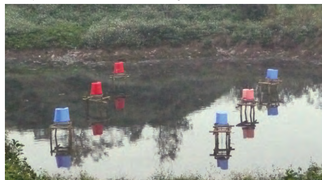
Installation of ECO-FAN completed in leachate adjustment pond (2012) *The ECO-FAN, made of waste materials, uses wind power to properly stir the pond.
