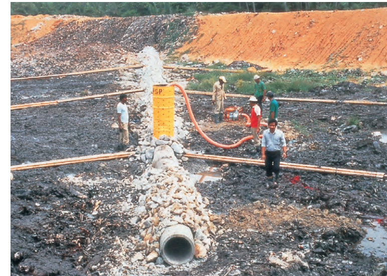
Recirculatory semi-aerobic landfill, using concrete pipe, bamboo and used steel drums
