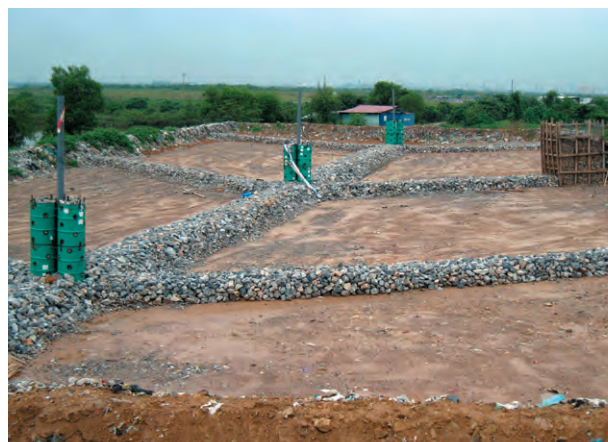
Ongoing improvement of landfill through the Fukuoka Method in Dinhvu, Hai Phong City (2011)
