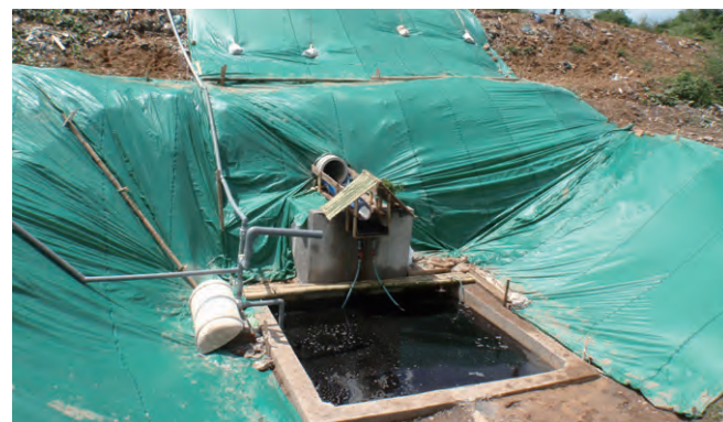
Tornado installed in leachate adjustment pond (2012) *The Tornado is a device that properly stirs the pond by creating whirlpools in the leachate and mixing air into the leachate.
