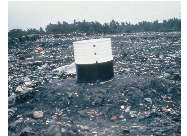
Gas ventilation system utilizing used steel drums
