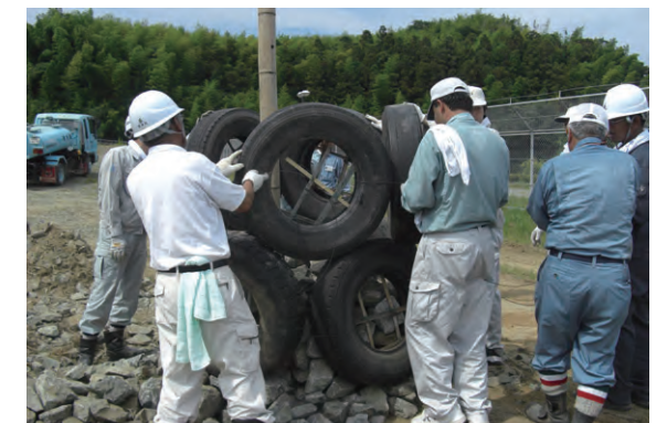
Practical training on how to install wasted tire-using gas collection and ventilation system (2008)
