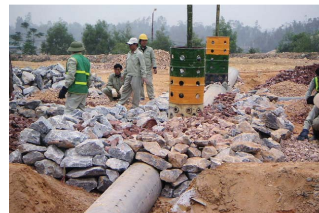
Installing gas collection pipe and ventilation system built from waste steel drums (Nam Son Landfill, Hanoi City, Vietnam) (2005)
