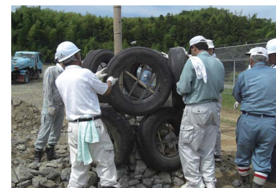
Practical training on how to install wasted tire-using gas collection and ventilation system (2008)
