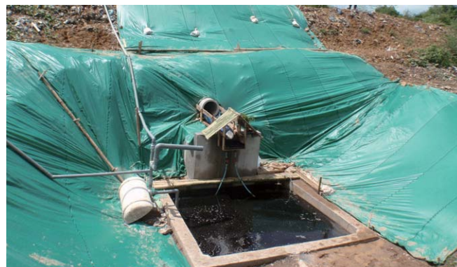
Tornado installed in leachate adjustment pond (2012)
