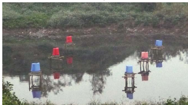
Installation of ECO-FAN completed in leachate adjustment pond (2012)
