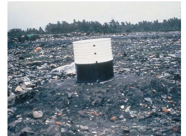
Gas ventilation system utilizing used steel drums
