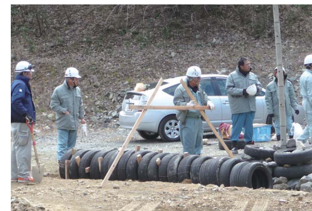
Practical training on installation of leachate collection pipes by use of waste tires.
