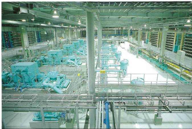
Uminonakamichi Nata Sea Water Desalination Center
